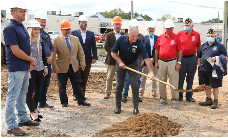
Craig Clabaugh, HART Center Executive Director, breaks ground at a ceremony on Wednesday, Sept. 16. He is joined by representatives from Conewago Enterprises Inc. and Bruce L. Jones Contractor Company as well as PA State Rep Dan Moul (fourth from left). Photo Credit: Darryl Wheeler, Gettysburg Times
